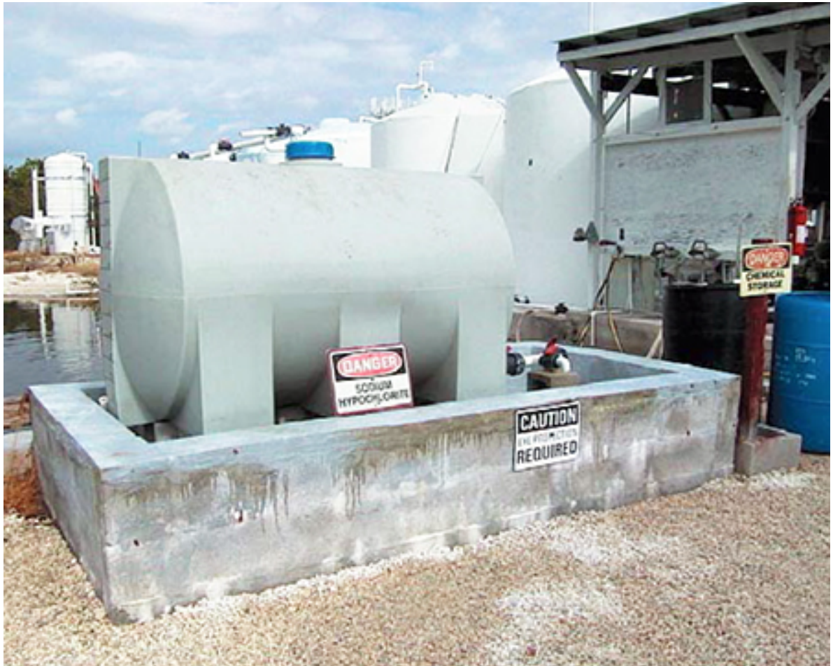
Secondary containment for chemical storage tanks minimizes the risk of accidental spills.
