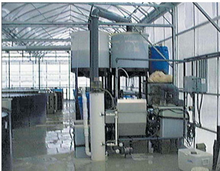
Biofilter complex at Target Marine in Sechelt, B.C. Canada.
