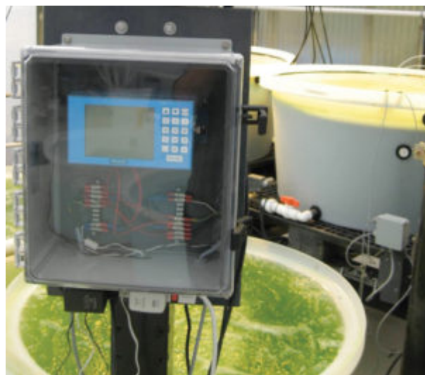
This HISTAR system controller has eight analog inputs and eight control relays.
