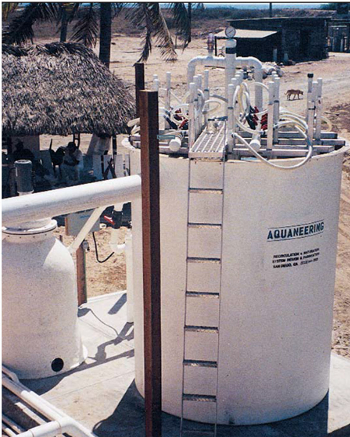
Fluidized bed biological filter with a flow rate of 15 liters/sec (200 gallons per minute).
