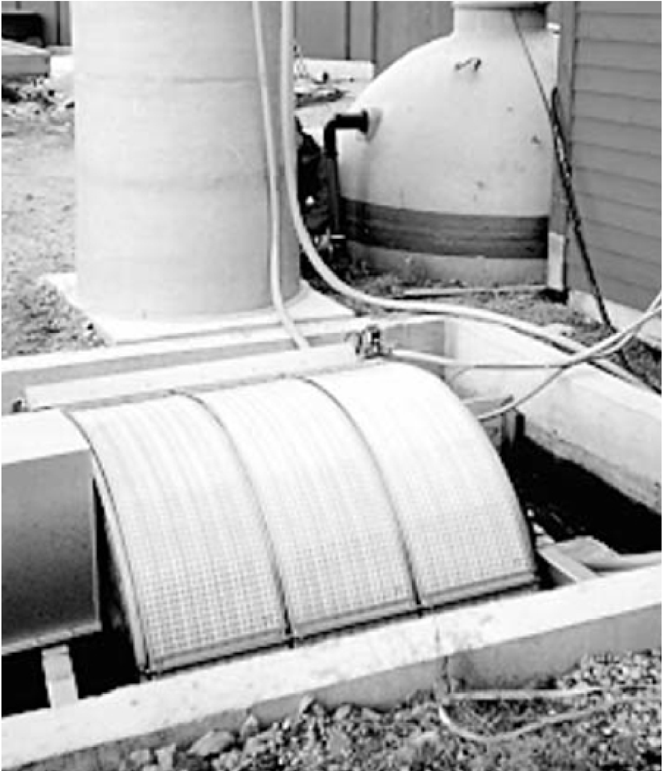
The effluent treatment system described at a hatchery in County Rogaland (Bokn Settefisk). The main units are a drum sieve, a thickening tank (tubular) and a unit for sludge stabilization.
