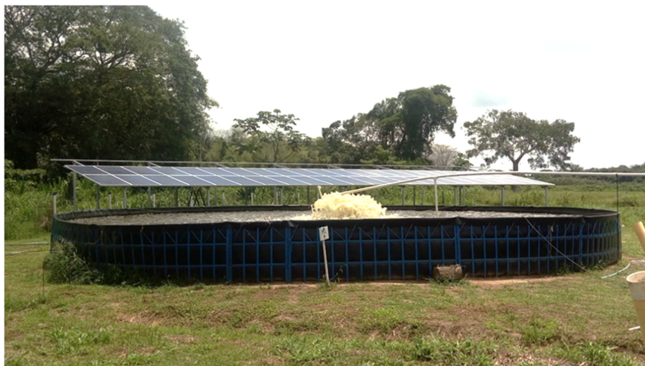
Fig. 1: View of an experimental production system used in the study, with high-density polyethylene (HDPE) geomembrane tanks and photovoltaic system.
