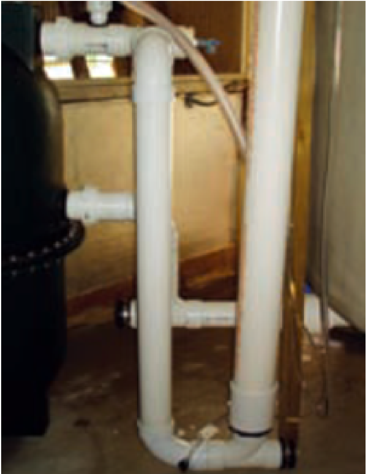
The clear pitot tubes behind the riser pipe indicate dynamic head losses when the biofilter clogs.
